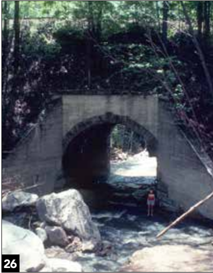
26 This very tall concrete and stone arch is on the Black Fork grade of the Western Maryland east of Elkins, West Virginia. My wife, at 5'-4", is dwarfed by the arch. We found debris apparently left by storm water high on the wing walls, illustrating the importance of culverts to protection of the roadbed. CJ Riley
